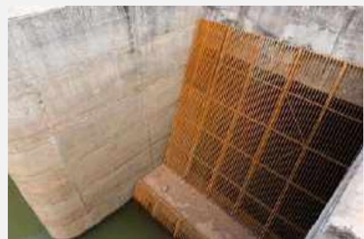
A typical trash rack
