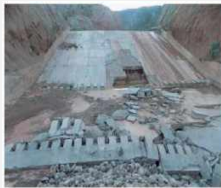
Damaged Stilling Basin of Domeli Dam
